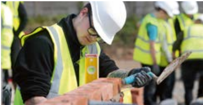
Left: Ten college students from Hugh Baird College, Bootle, visited Persimmon's Edinburgh Park Development in Liverpool, learning about bricklaying and gaining hands-on experience of an operational construction site.
