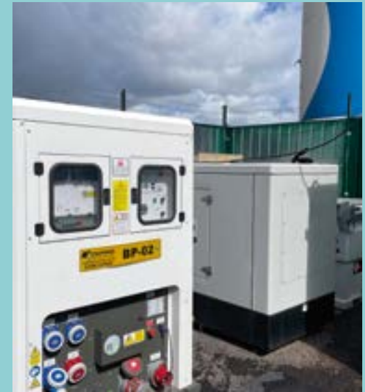
Above: Hybrid generator trial at Llanwern, East Wales.
